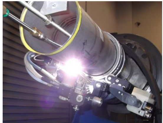
Figure 1: Orbital GTAW Welding a 4 in. Schedule 10 Pipe Specimen in the 5G Position
